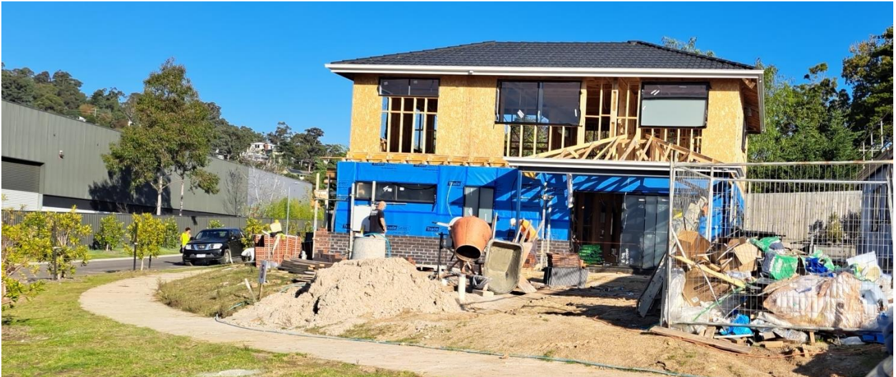
2 Wynnlea is another double storey dwelling constructed with BV and having a pitched hipped tile roof on a compact allotment within the subdivision.
