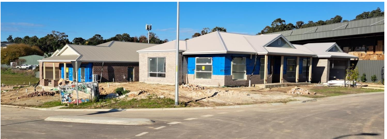
1 and 3 Janson place are currently under construction and are single storey BV dwellings with steel roofs. To the south, behind, these dwellings another Commercial Zone2 dwelling can be seen.
