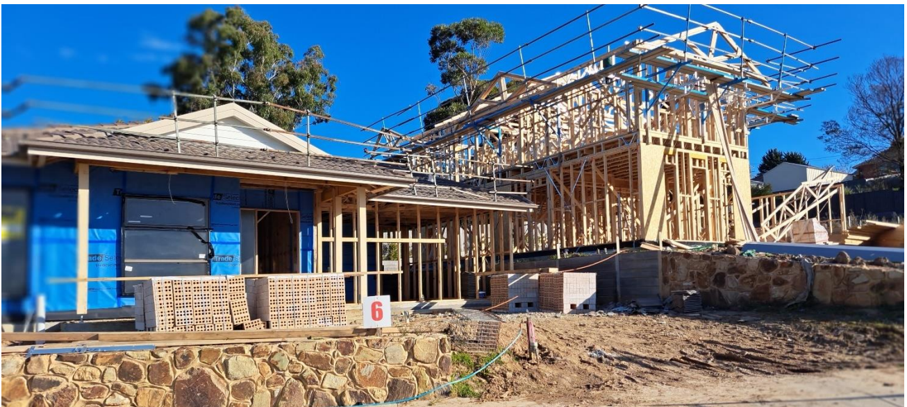
4 Wynnlea (to the left) and 1 Potters Rise dwellings under construction above. 4 Wynnlea is a single storey BV dwelling with pitched tile roof with a Dutch gable feature while 1 Potters Rise is a double storey dwelling.
