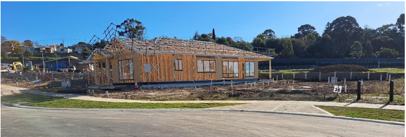
8 Janson Court near the subject site is under construction and will be a single storey dwelling.
